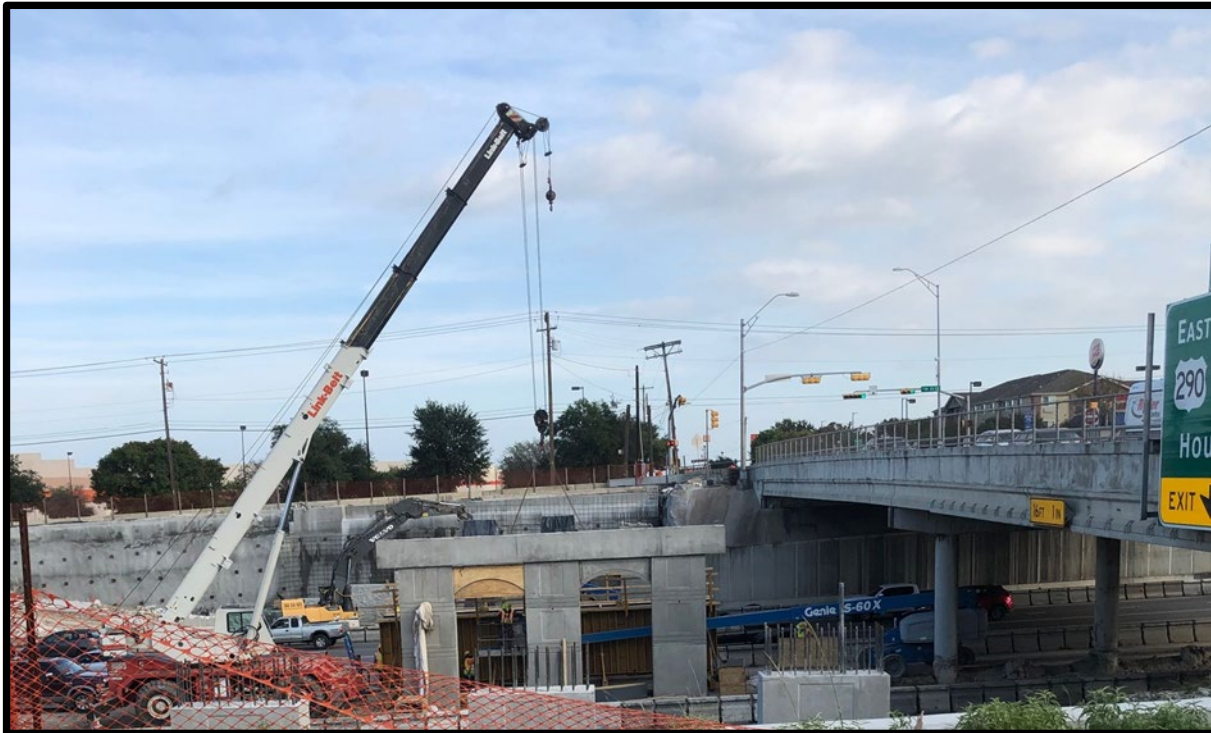
Completed Bent 3 cap in the center of I-35 for the St. Johns south to north U-turn bridge
